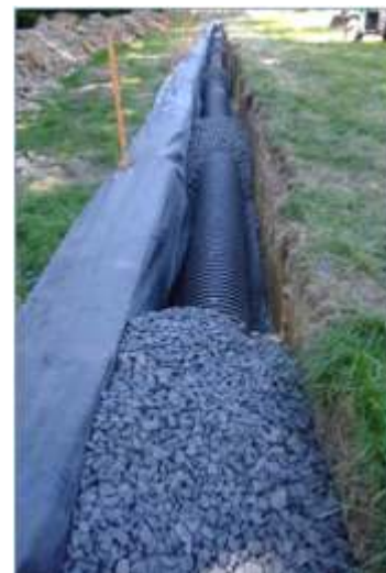
French drains at North Wyke use perforated pipes to capture and funnel water to special flumes. Image: North Wyke
